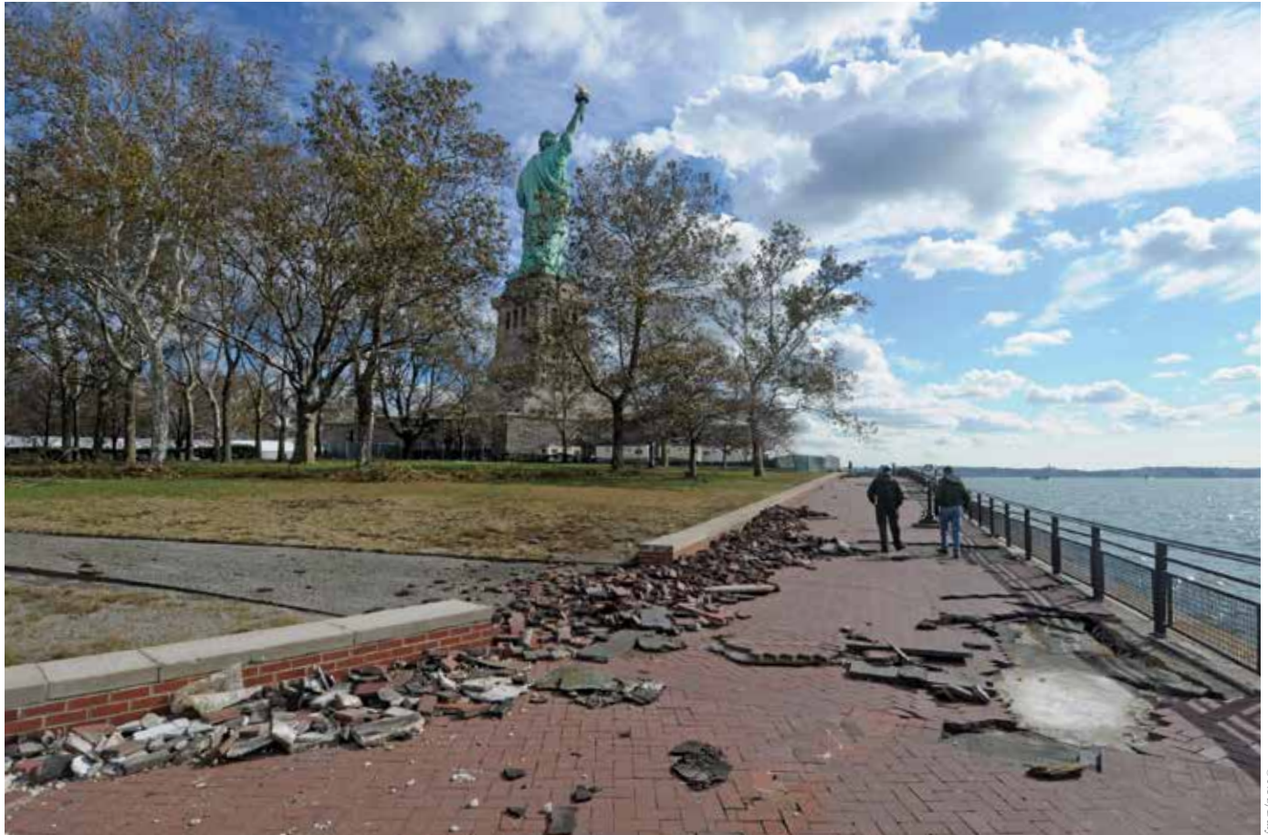
Hurricane Sandy's massive storm surge destroyed most of the radio equipment, electrical infrastructure, and security systems of both Liberty and Ellis Islands. Floodwaters inundated three-quarters of Liberty Island—some of the aftermath is pictured, above—and the beloved landmark was closed to the public for more than eight months. 34
