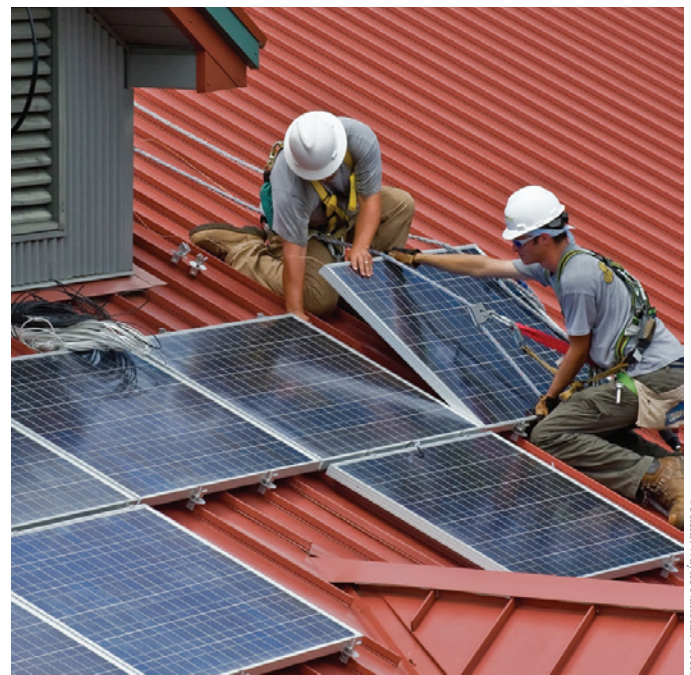
Workers install PV panels on a national forest facility in southeastern Ohio. Solar systems grace a rapidly growing number of houses, office buildings, parking structures, schools, and churches.
