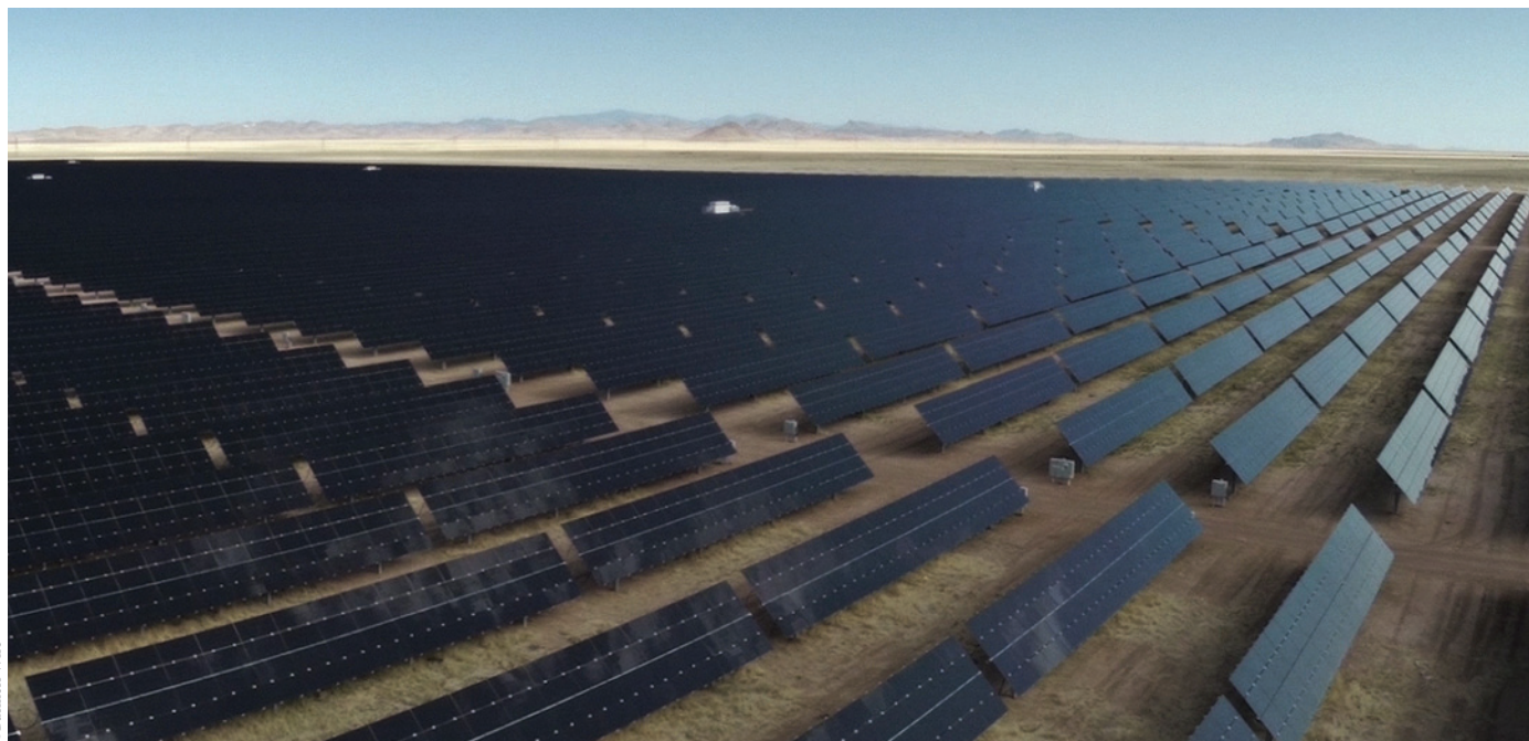
Large-scale solar is an important part of moving the electricity sector away from fossil fuels and their many negative consequences. The 50 MW AC Macho Springs solar project, owned by Southern Power and Turner Renewable Energy, is the largest solar facility in New Mexico, a state with an increasing amount of solar and other renewable energy generation helping the power sector address global warming and other issues.
