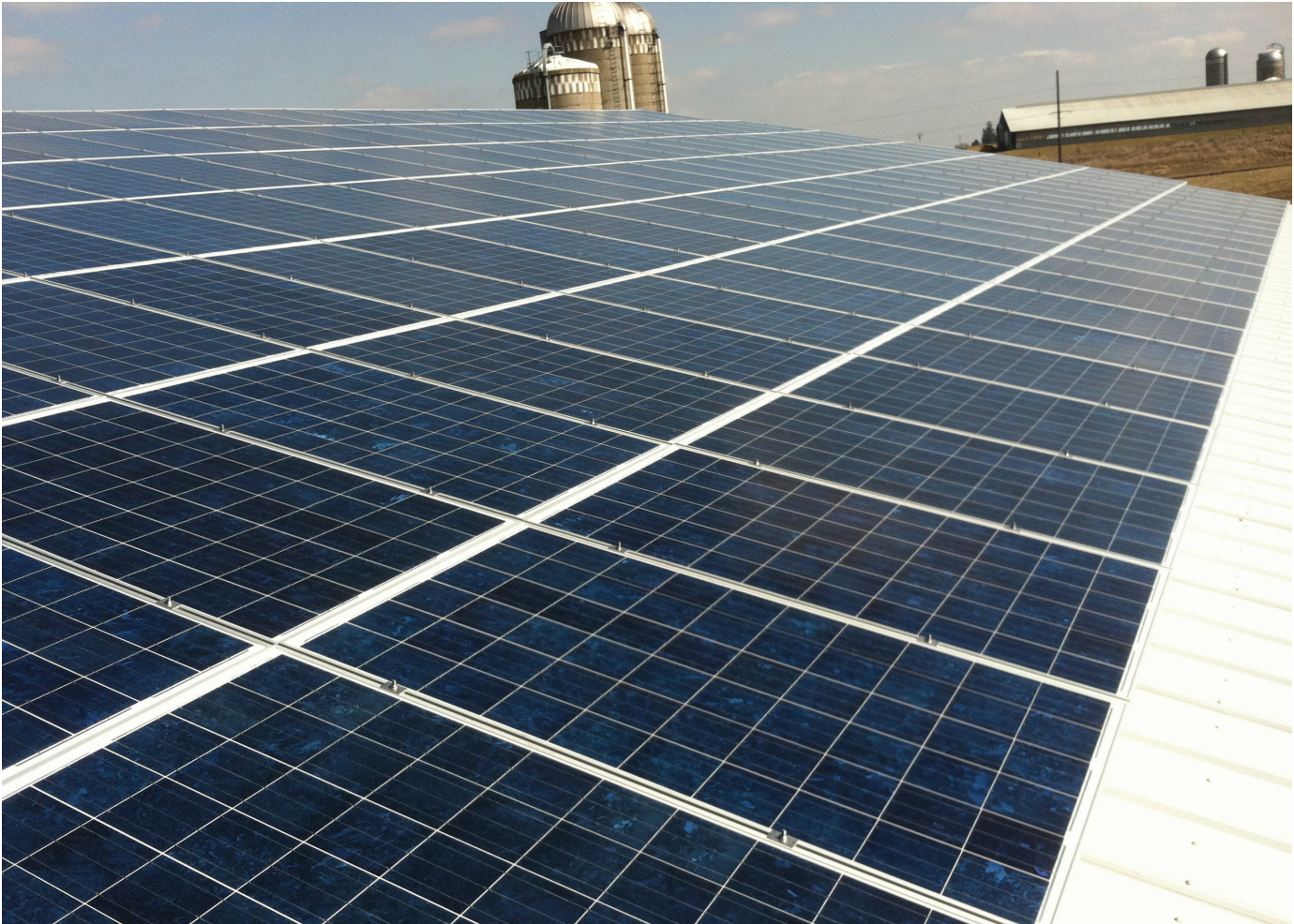
In 2012, Gibbs Dairy, in southeastern Minnesota, installed 166 solar panels that are expected to supply the farm with 30 percent of its electricity needs annually.
