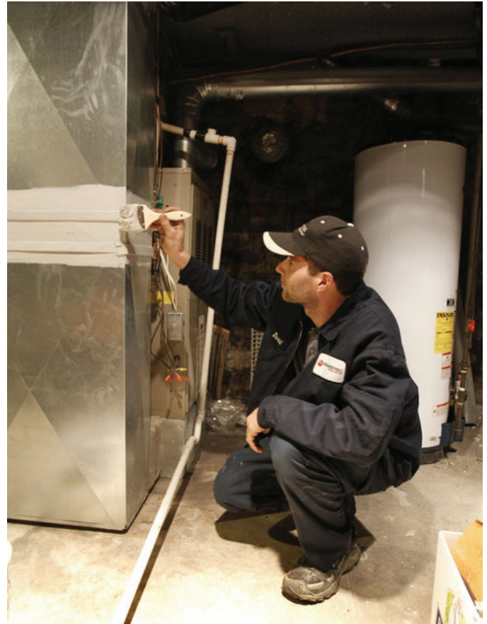
A technician seals ductwork in a home in Lexington, KY, following an energy efficiency audit done in partnership with the KY Home Performance program. In addition to providing rebates for energy audits, the program offers financing to pay for identified energy efficiency retrofits that are achieving average energy bill savings of 26 percent (Sloan 2012).
